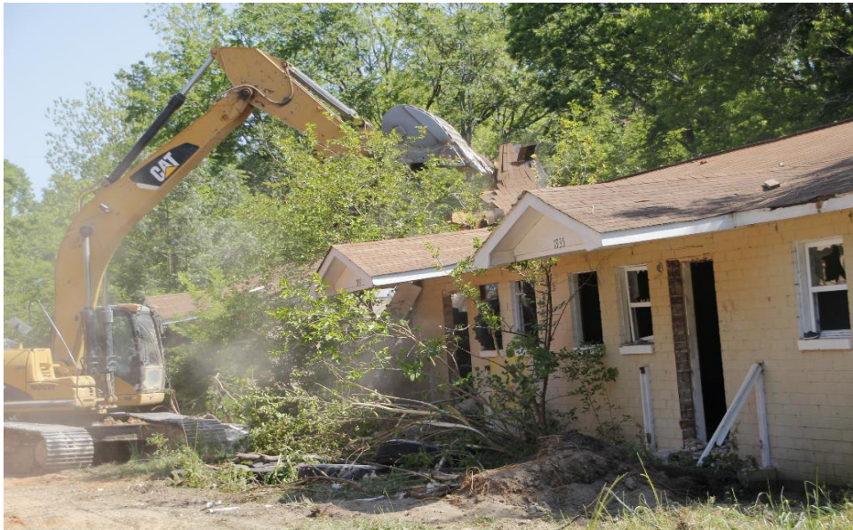
Demolition from another angle of Houses on Moore Street in May of 2012
