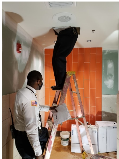
Inspector Mullis and Inspector Rembert. Inspector Mullis inspecting the sprinkler system at Burger King.
